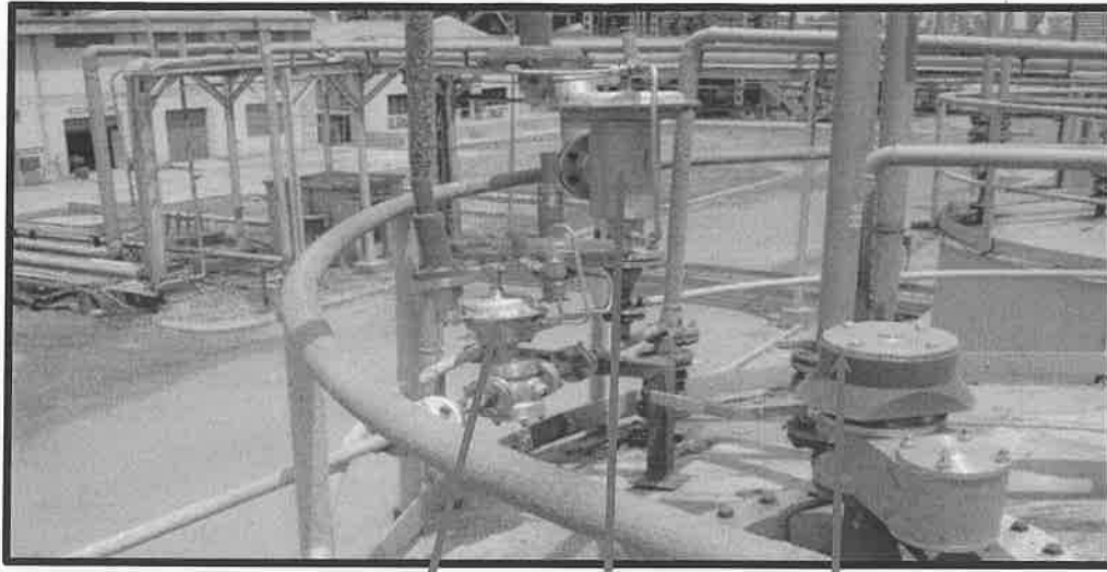
PRV for N2 SRV for N2 Breather Valve Blanketing Blanketing Nitrogen Blanketing System On Storage Tanks
