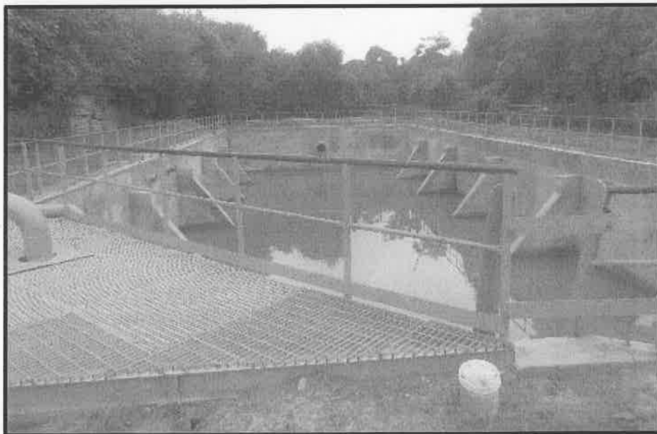
Surface water run-off collection pit
