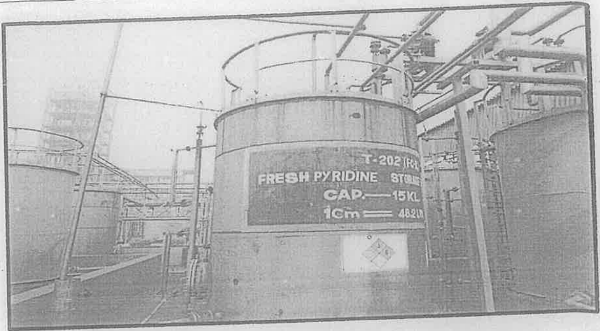
Chiller attached to vent of fresh pyridine Storage tank at CPC plant.
